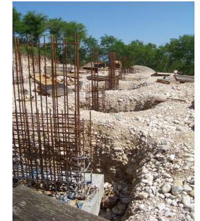
The rebar ties, the dirt moved, the concrete mixed all by hand.
